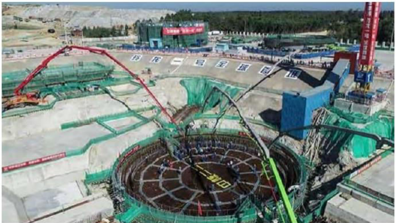
China advances in nuclear power with world's first small modular nuclear reactor Photograph:( Twitter )
